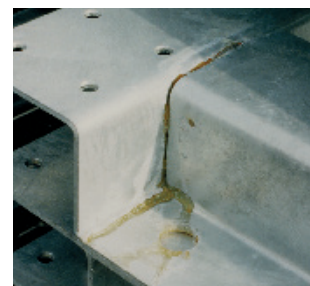
Discoloration caused by acid trap.
